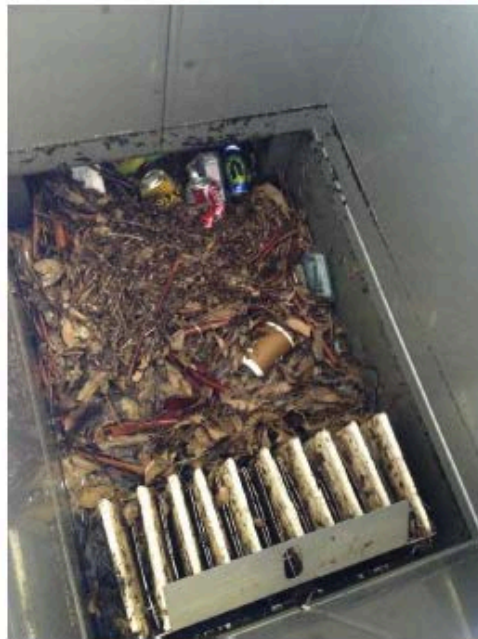
Figure 9: Gross Pollutant Testing
