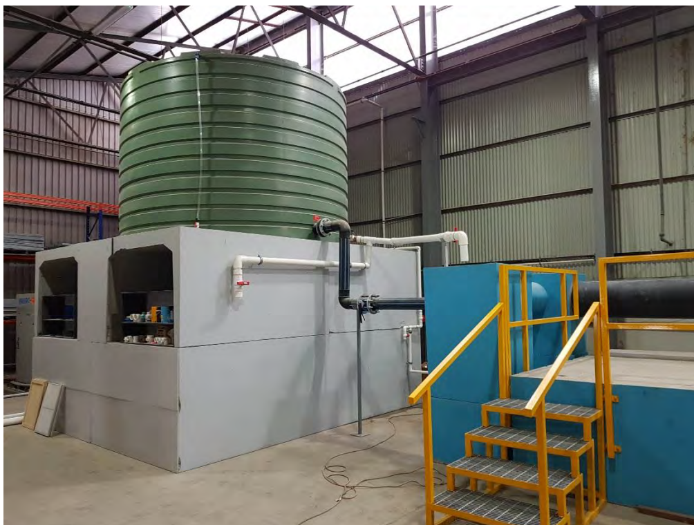
Figure 2 - Photograph of the oil/water separation test setup, showing the inflow water storage and inflow pipework
